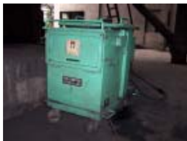
100 litre per hour On-line Electrostatic Liquid cleaning machine in operation
